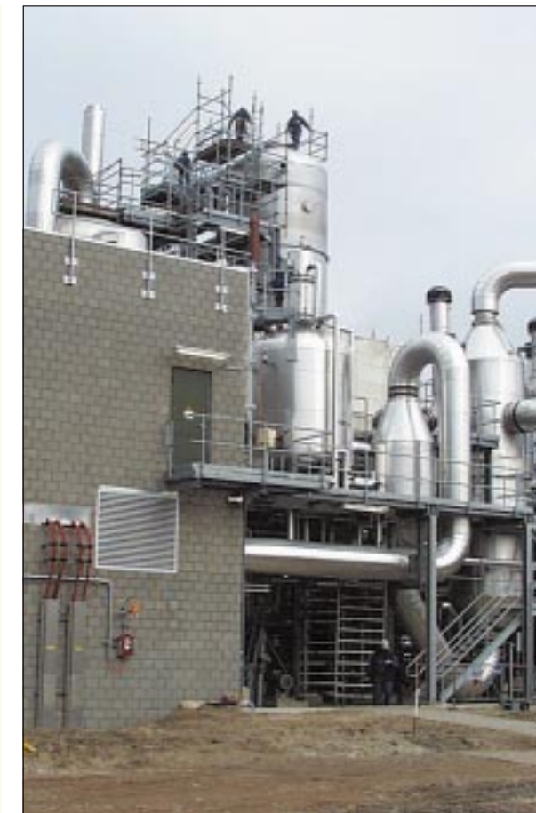
The final touches on the huge (over 250,000 tpa) new plant for DuPont.
